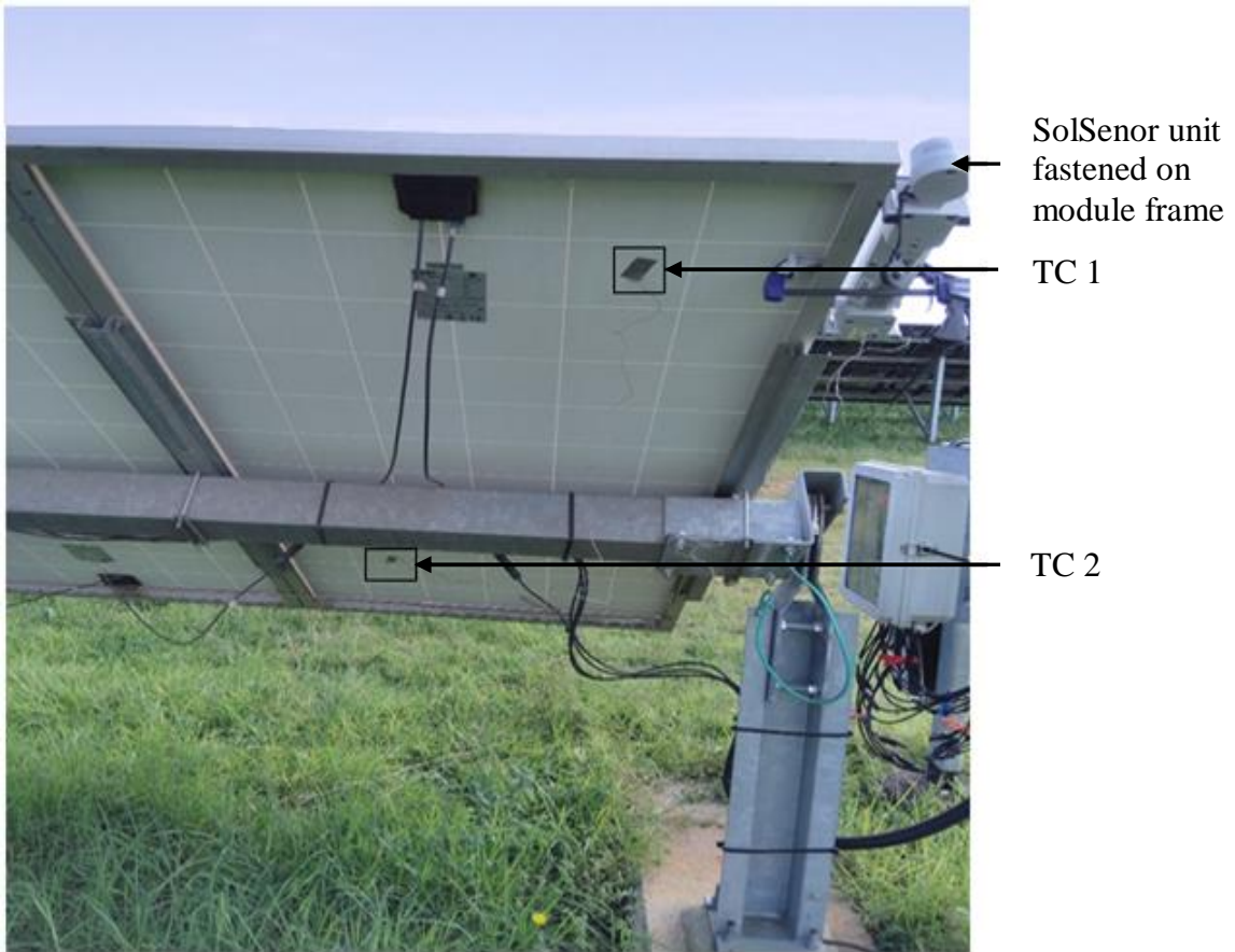
Figure 3-6: Type K thermocouple tips stuck diagonally on the backside of a PV module and a SolSensor unit at same inclination angle as the modules.
